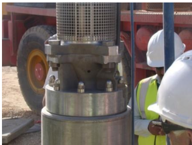
Pump Installation initiated after clearance from Commissioning (Motor water filling, IR value, winding resistance & RTD Checks)
