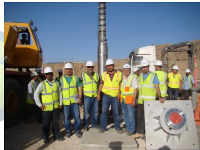
Pump Installation completed. Piping & Valves installation & cabling completed and ready for Commissioning
