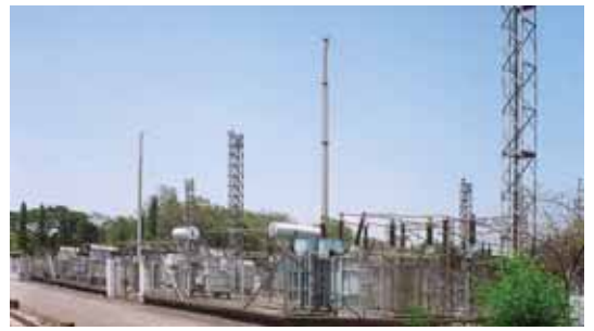
▲ Substation & Telemetry, Panjarapur, Mumbai
