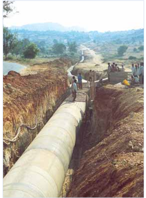
▲ Water Transmission Line, Bangalore
