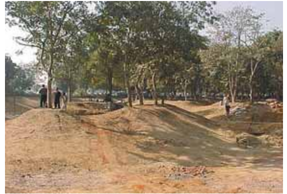
▲ Rain Water Harvesting, Maruti Udyog Limited, Gurgaon ▼
