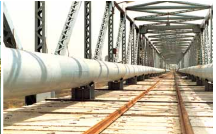
▼ Raw Water Transmission Lines, Ahmedabad
