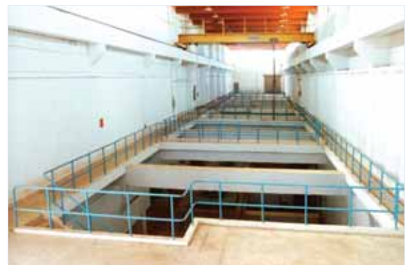
▲ Terminal Sewage Pumping Station, Ahmedabad
