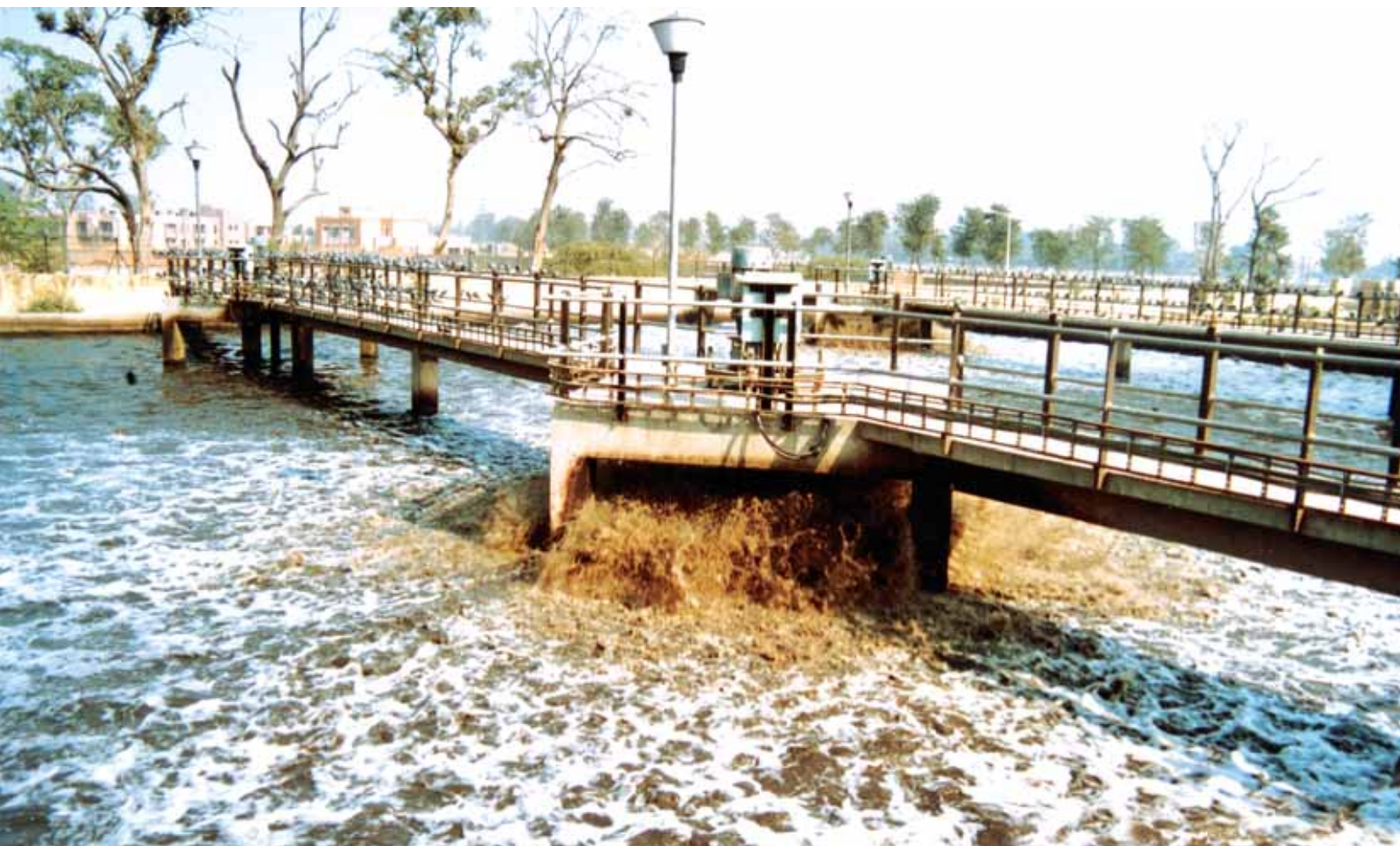
▼ Aerators at Yamuna Vihar Waste Water Treatment Plant, New Delhi
