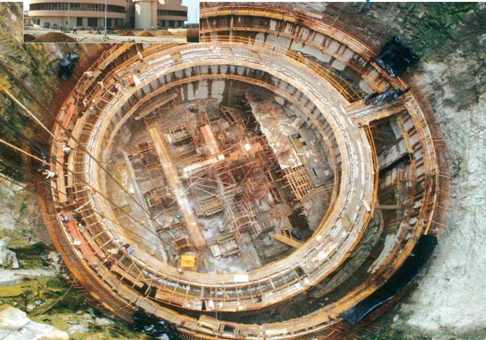
◀ 1900 Mld Influent Pumping Station, Bandra, Mumbai
