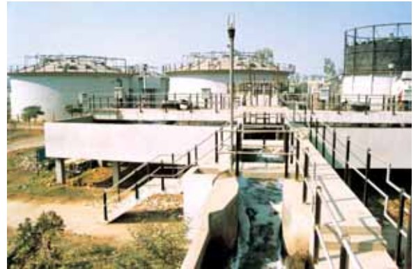
▲ Digestors & Gas Holder, New Delhi
