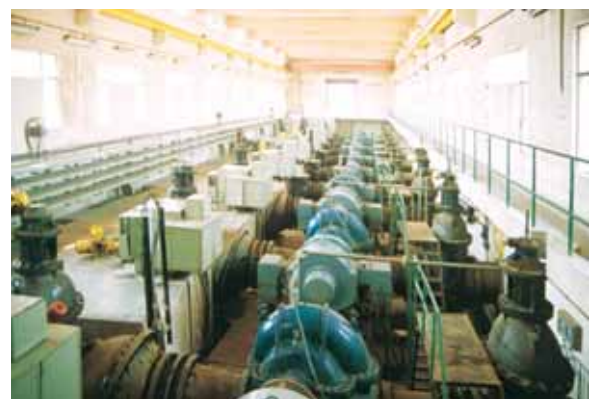
▲ Sludge Pumping Station, Kondli, New Delhi
