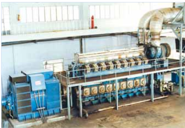
▲ 6.5 MW Diesel Generator Set, Chemplast Sanmar, Mettur
