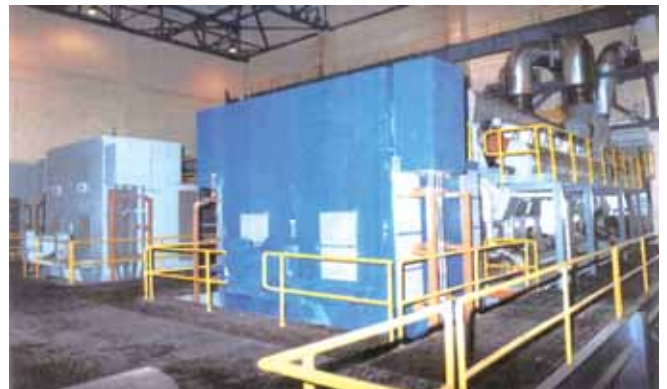
▲ 3 x 9.6 MW Diesel Generator Sets, Kudremukh Iron Ore Company Limited, Mangalore
