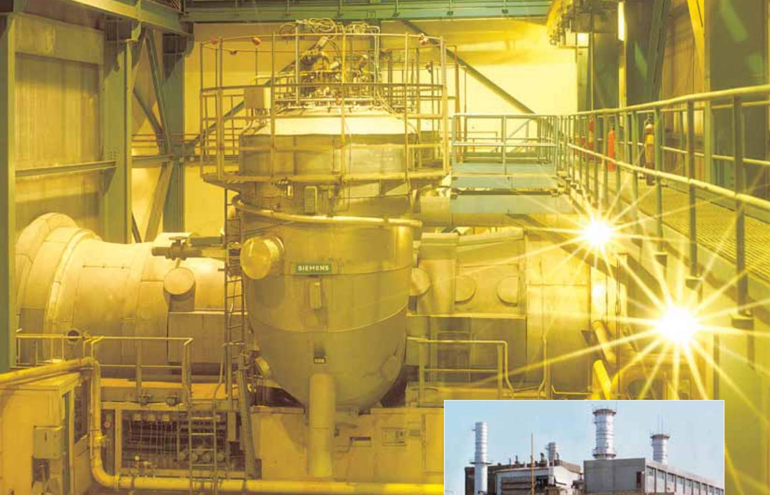
▲ Siemens V94 gas turbine 205 MW CCPP, Trombay
