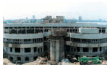
Influent Pumping Station, Mumbai
