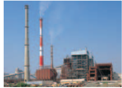
2 x 120 MW Thermal Power Plant, Jojobera
